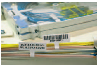
Fibre optic cable markers
