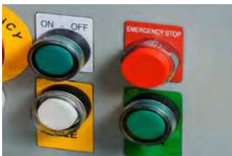
Control panel labels
