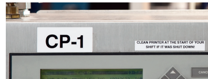
Control panel & electrical panel labels
